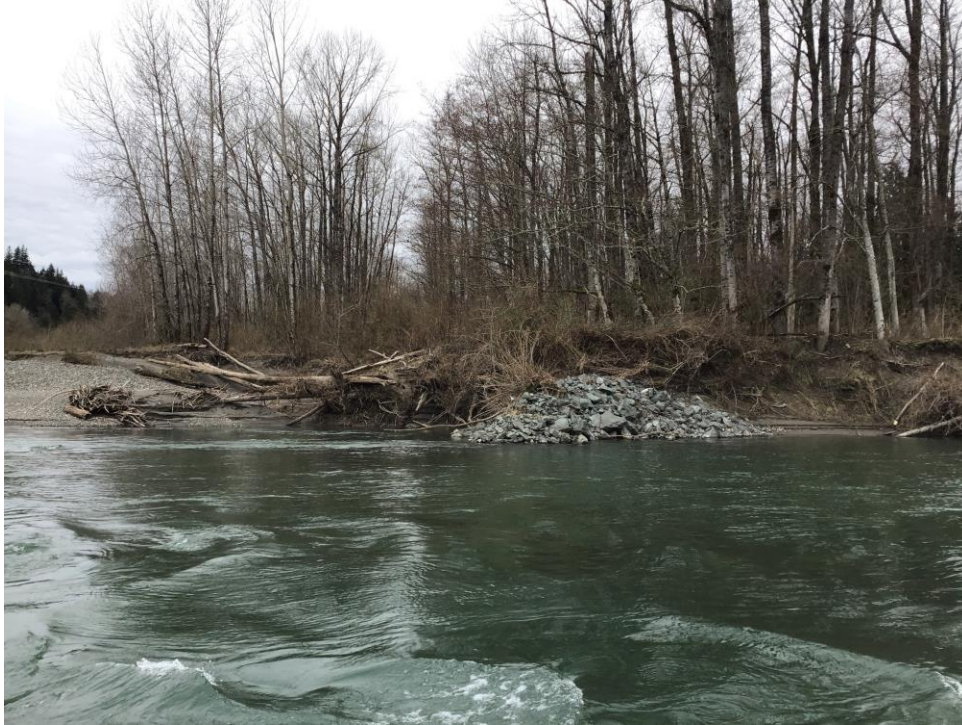
Figure 3. Skiyou bank rock on right bank. Flow direction from right to left of photo. Scour and undermining of the streambank is visible around the rock.
