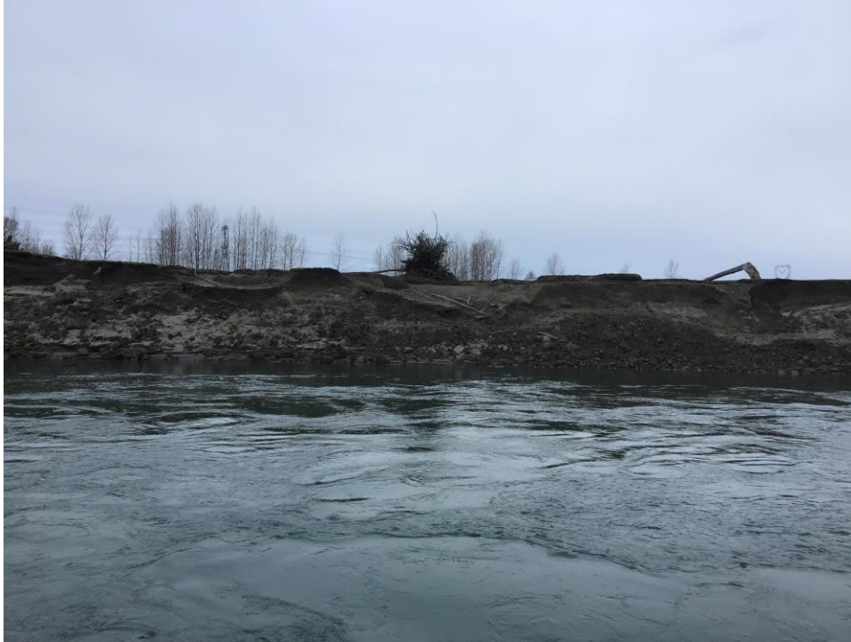
Figure 9. Right bank of the Skagit River immediately along the Benson parcel and evidence of active erosion, located upstream of Skiyou rock. Flow direction is from right to left of photo. Note that trees on the bank are deposited from recent flood flows (personal communication with Emily Derenne, 2020). Power transmission lines are visible in the background of photo.
