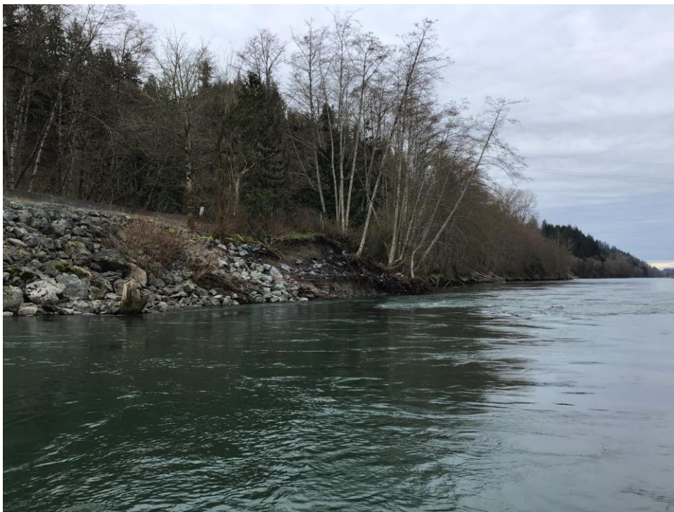
Figure 6. Left bank along South Skagit Highway, view looking in the downstream direction. Riprap is visible in the foreground. Active erosion of the streambank was observed downstream of the revetted bank. Shown in the center of the photo is old wood embedded in the streambank, which has been exhumed by the eroding bank.
